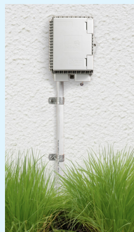
nbn utility box mounted on the surface of an external wall
