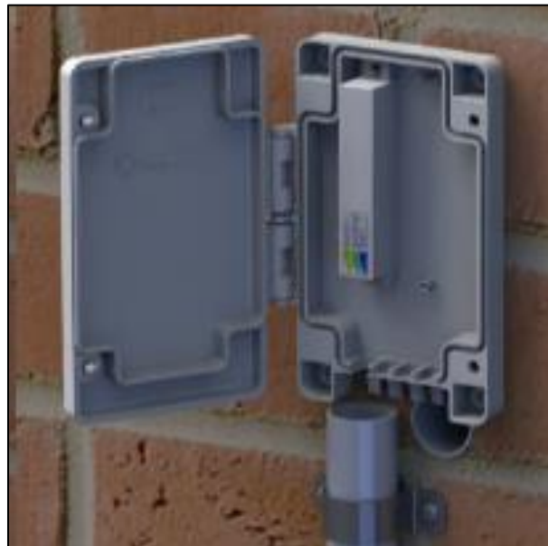
Figure 14. nbn™ NTD with VDSL2 centralised filter installed
