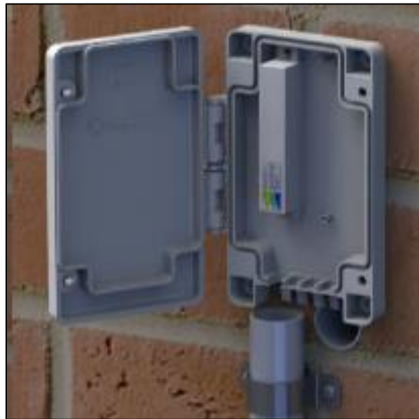
Figure 14. nbn™ NTD with VDSL2 centralised filter installed
